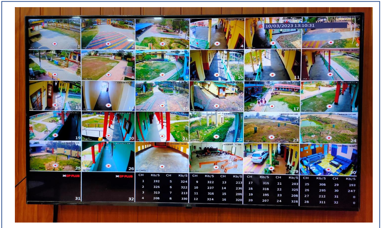
Live display of the CCTV Camera
