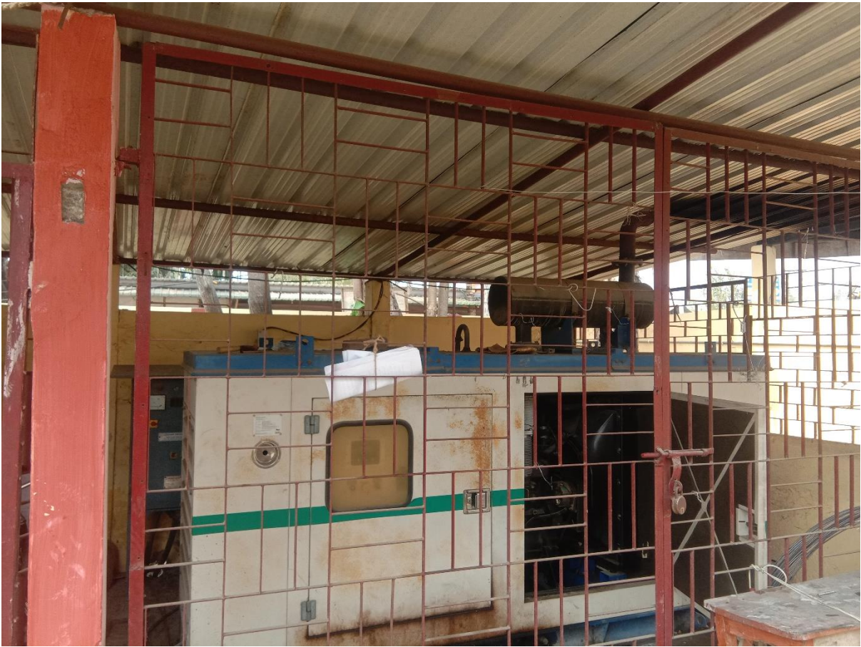
Photo of Generator Room
